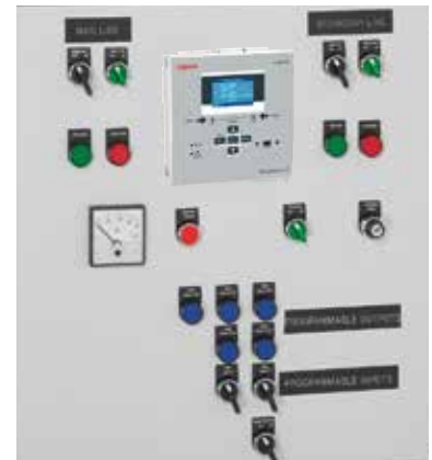
Control panel of a supply inverter with automation control unit Cat. N° 4226 80
