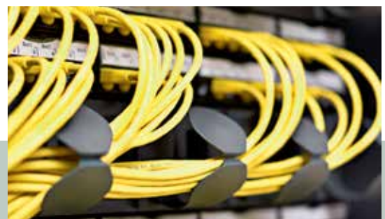
Patch panel (p. 78, 83, 87, 88, 92)
